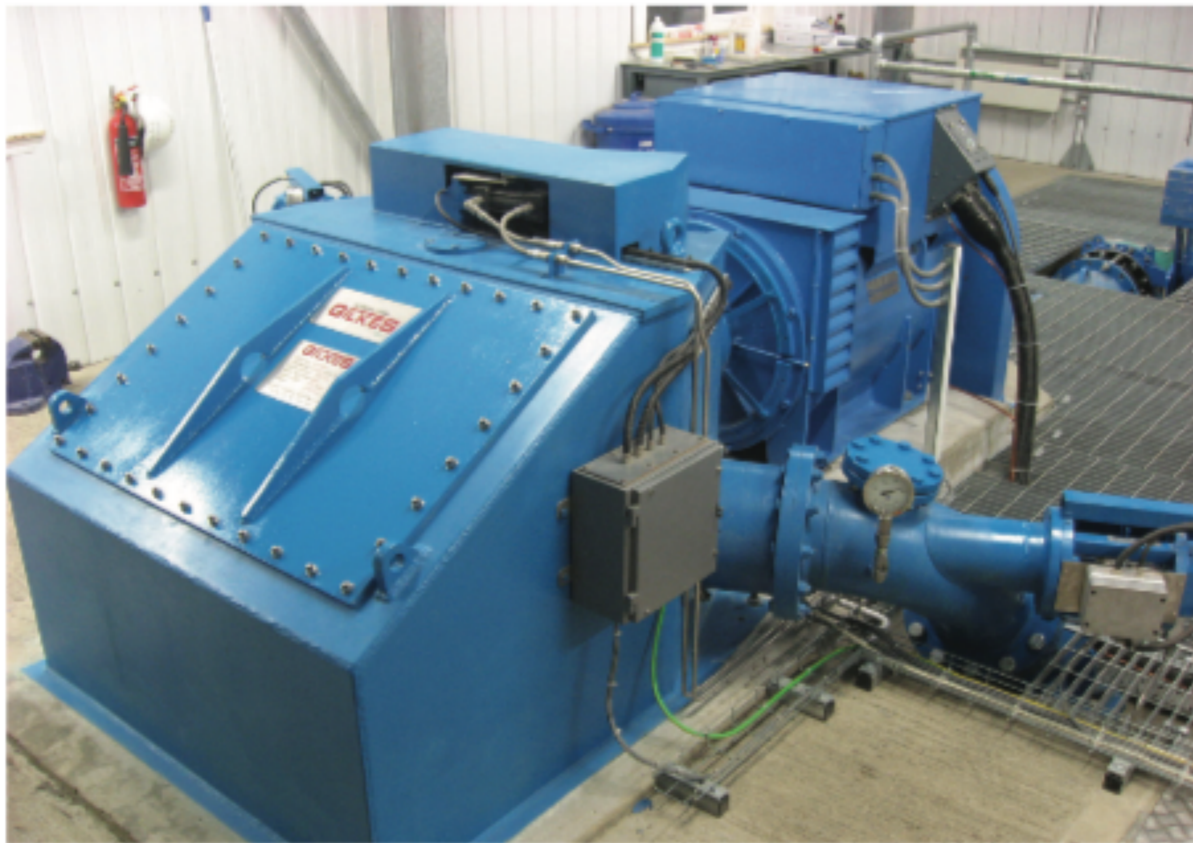
Gilkes Turgo installed.
