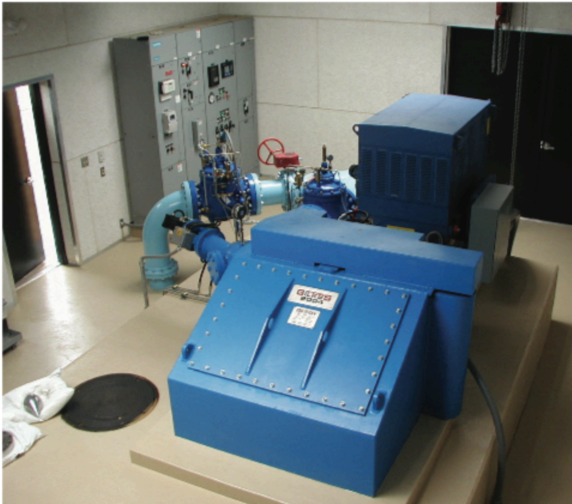
12 Inch mean diameter singlet jet Gilkes Turgo installed at Draper Irrigation Company, UT, USA. Net Head 633ft, Rated Flow 11.7cfs, Speed 1800rpm, Power 511kW, Year 2004
